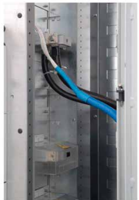
CABLE COMPARTMENT VANO CAVI
